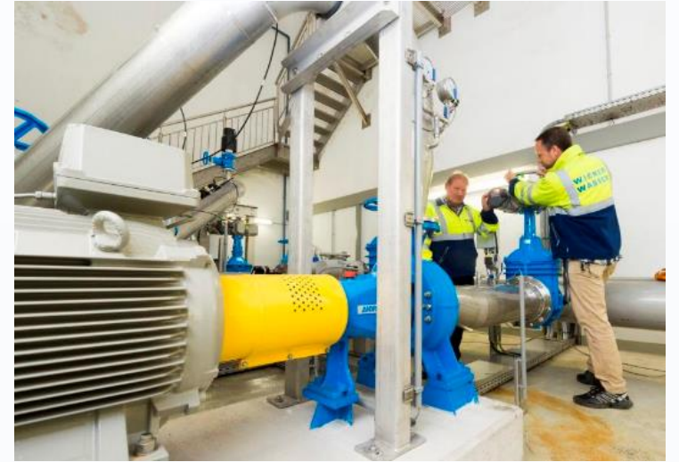
DWPP, Service chamber, Reservoir Schafberg (2017, 100 KW)
