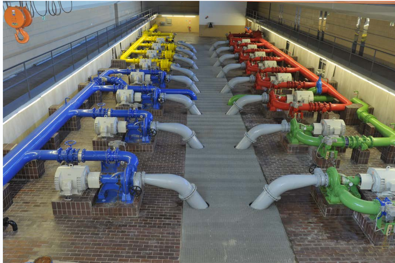
Pumping Station Laaerberg
