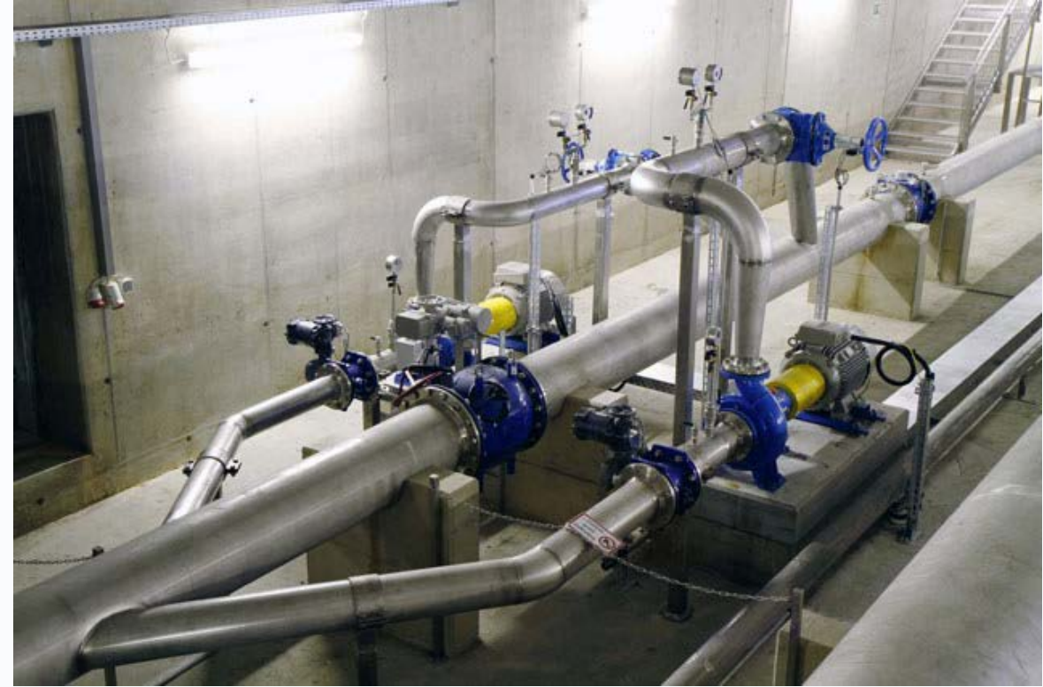
DWPP, Service chamber, Reservoir Wienerberg (2013, 65 KW)
