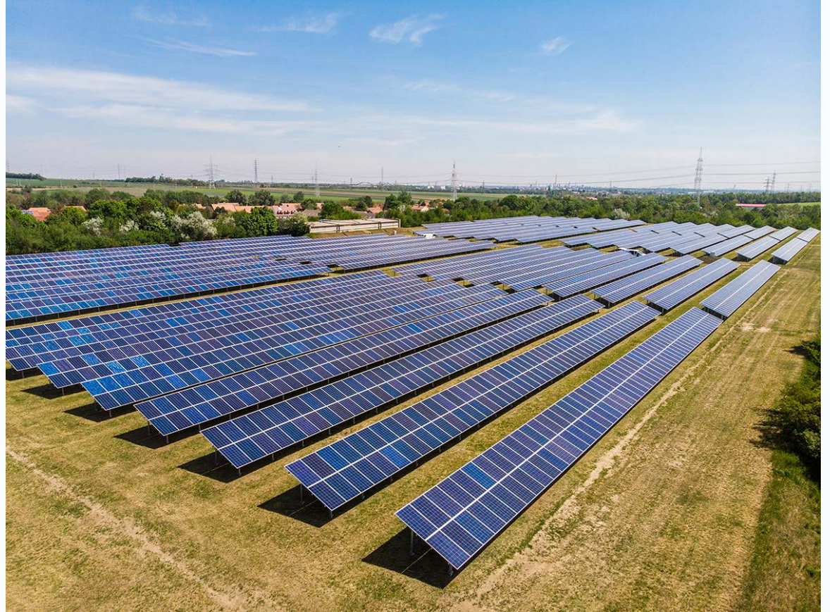
PV power plant, Reservoir Unterlaa, (Vienna Energy 2020, 2 MWp)
