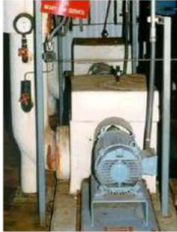
Combined motor & pump efficiency = 59%
