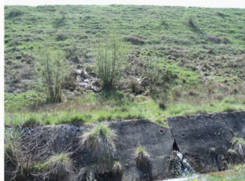
Seepage springs and slope instability
