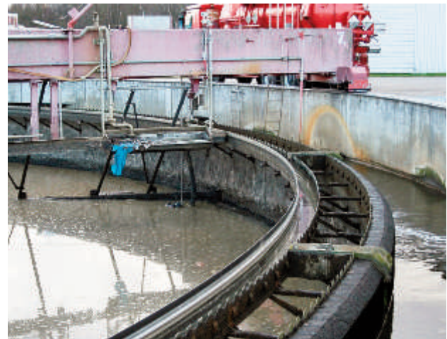
Photo 2: Wastewater treatment plants with plastic bags in a sedimentation tank (plant revision).
