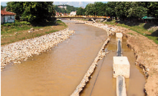
A new water supply pipeline in Valjevo was seriously damaged
