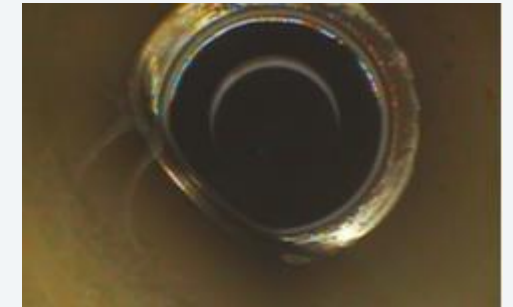
Service connection without illegal connection
